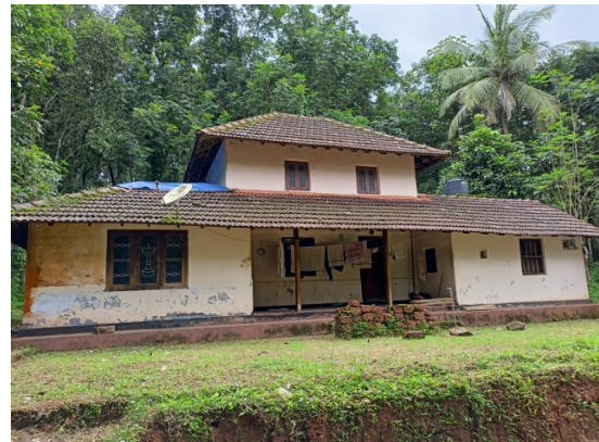
One of the affected House
