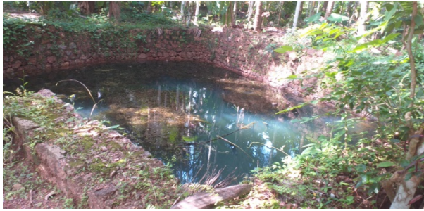
Affected Nagathankotta Pond
